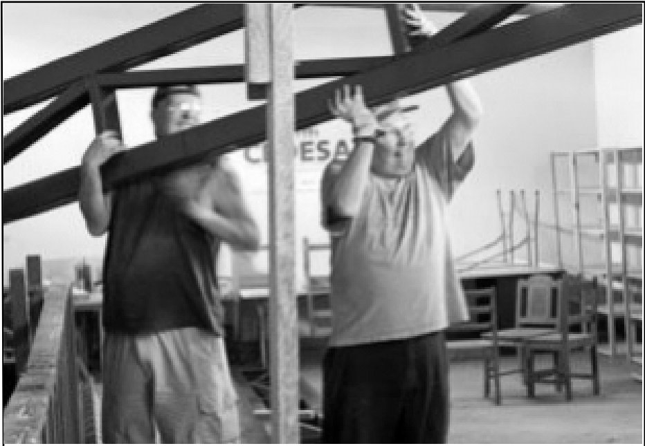
John Cambronne and Donald Meese had their hands full on this beam installation at the remodeled Jalapa Public Library. Photo by Lisa Fitzgerald
